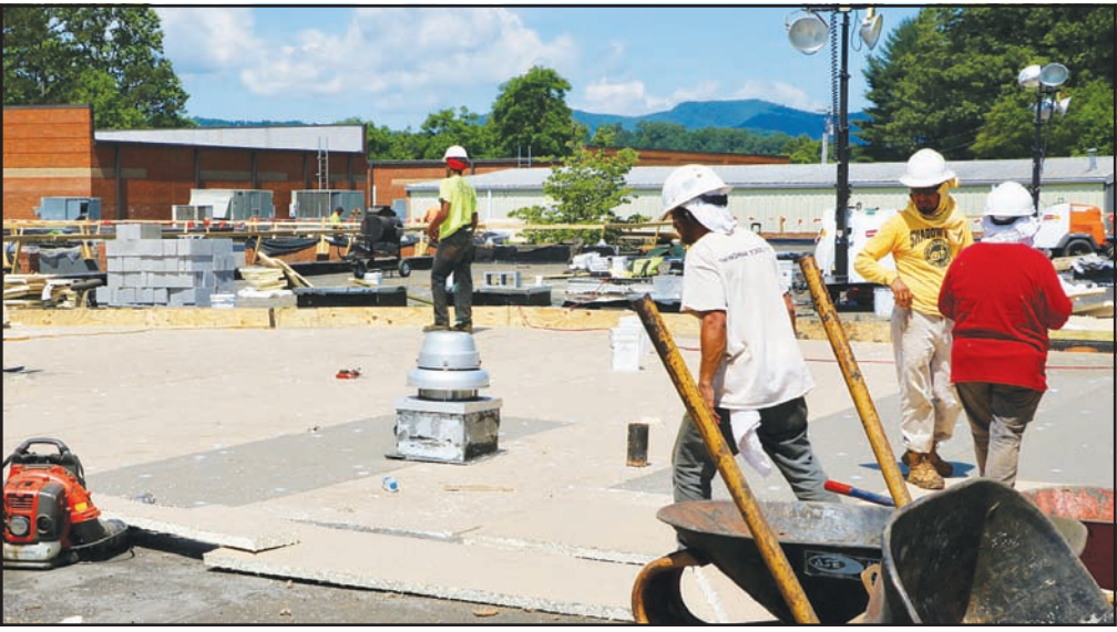
Workers installing the new roof on the joint middle/high school building of Towns County Schools in June 2018.
